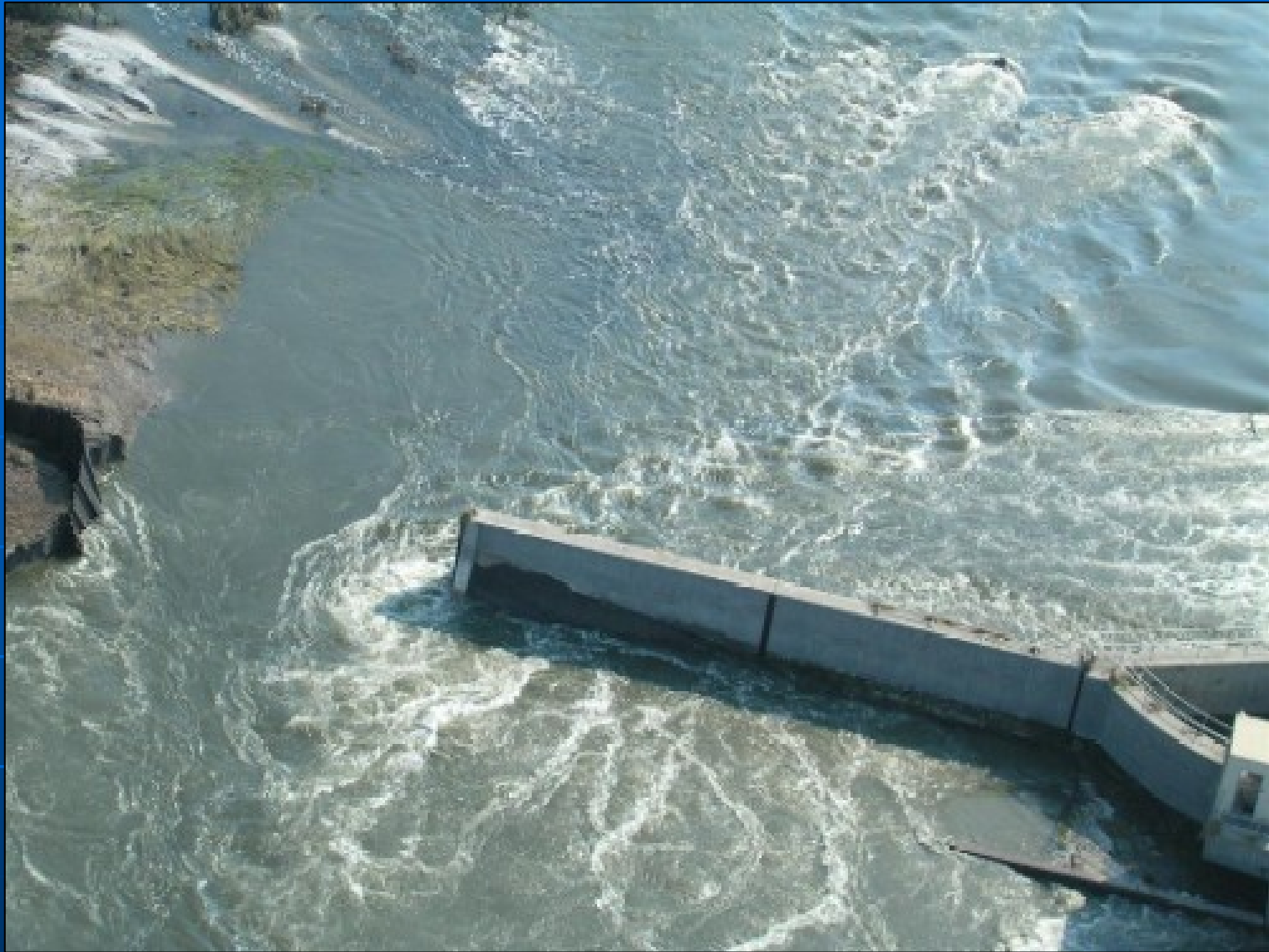
East Side IHNC North Breach, near Florida Ave. bridge and pumping station, during inflow. Note narrow chasm defined by this failure and dramatic flexure of the sheetpiles.
